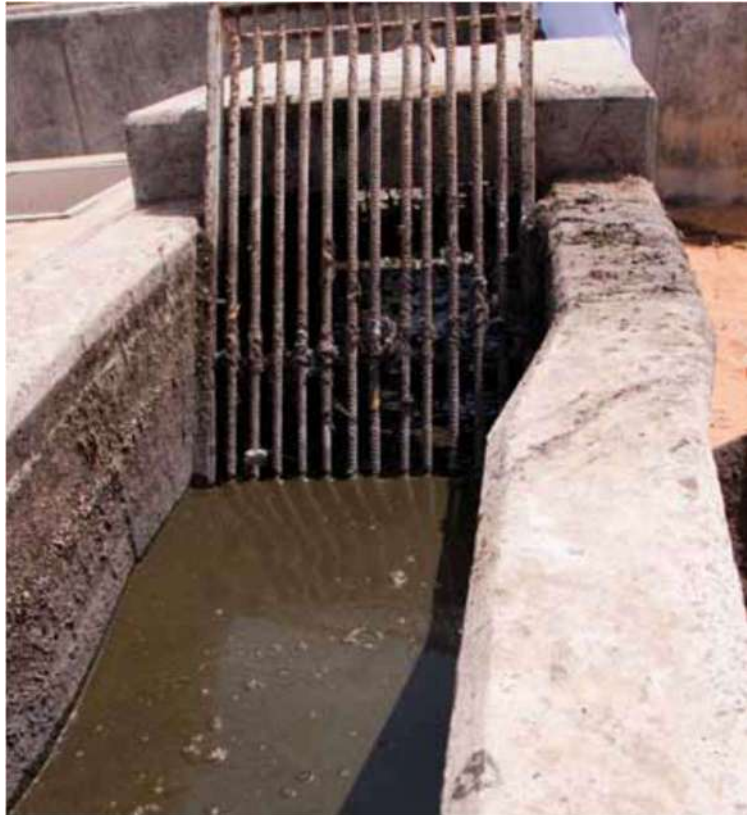
Fig 2: A typical manual screen channel in the septage plant. (Source: Linda Strande)
