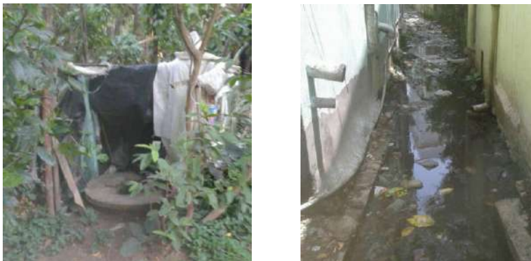
Figure 4-3: -Pit latrine and septic tank outfall discharging into open drain
