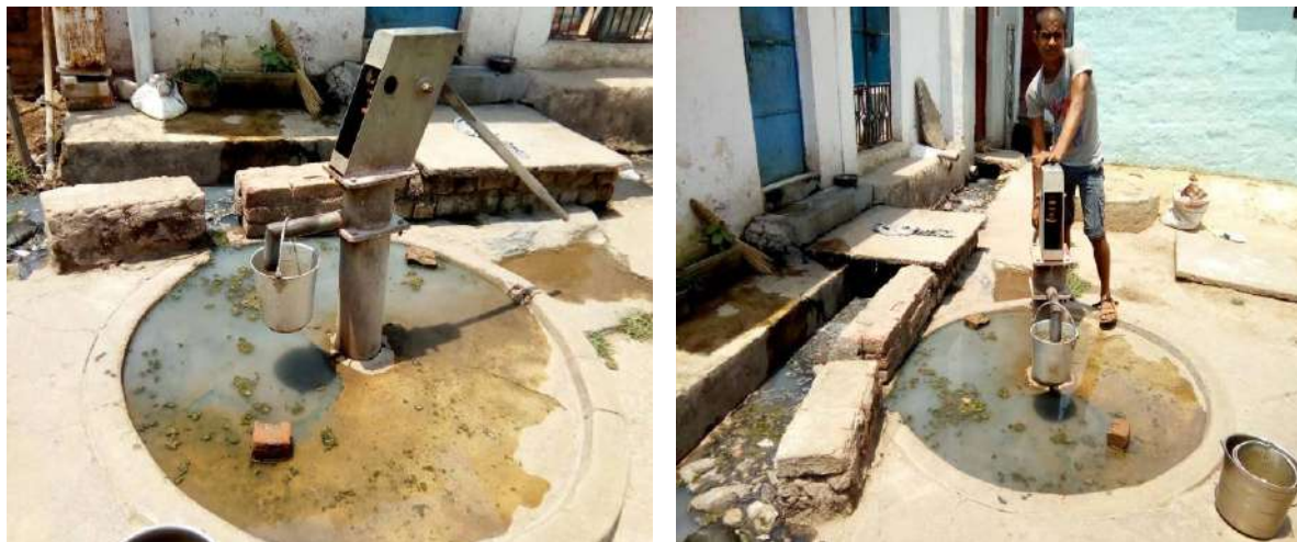
Figure 4-3: -Drain water overflowing near the outlet channel of hand pump in Bondamunda
